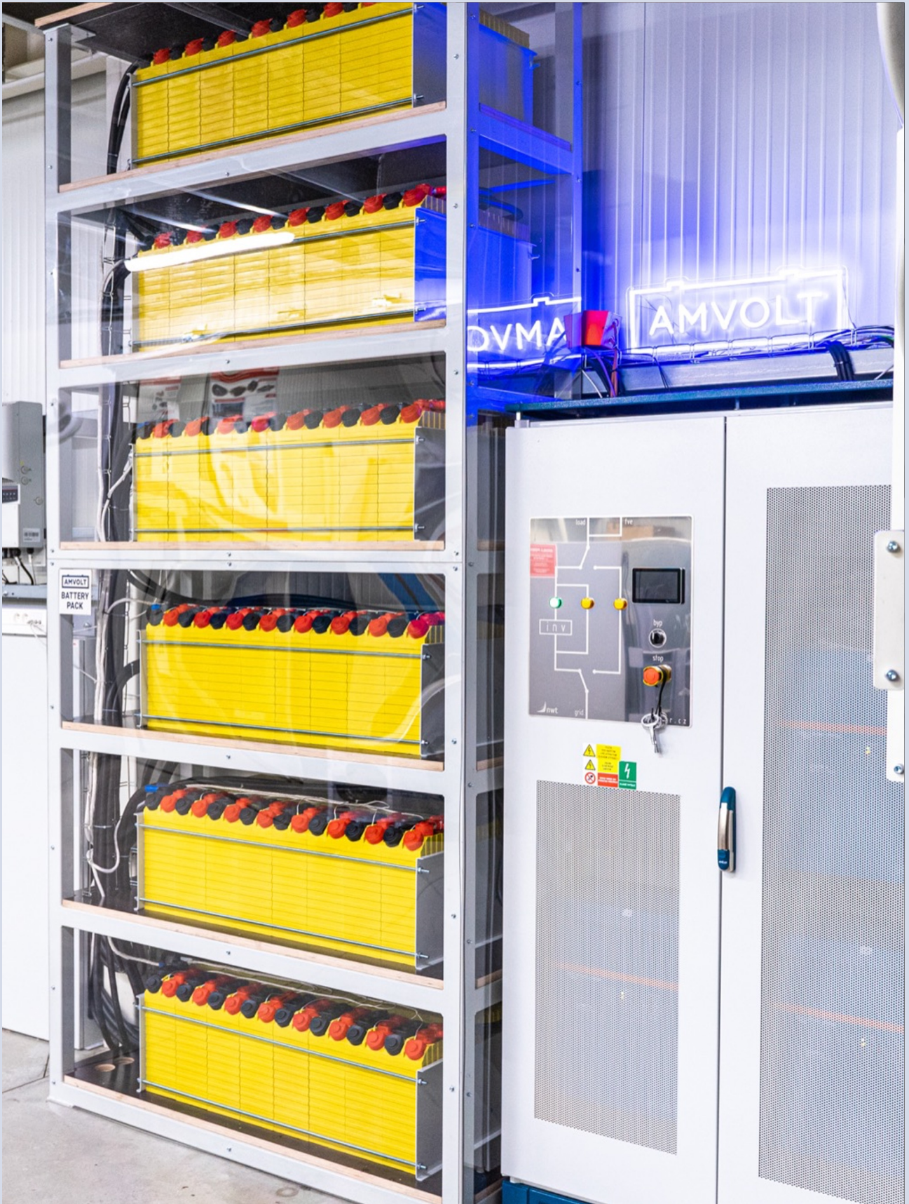
Fig.: Example of dimensionally modified AMVOLT 50kWh LV Modules according to customer's specific space requirements, installation partner Tomáš Vocilka (Asolar s.r.o.)
