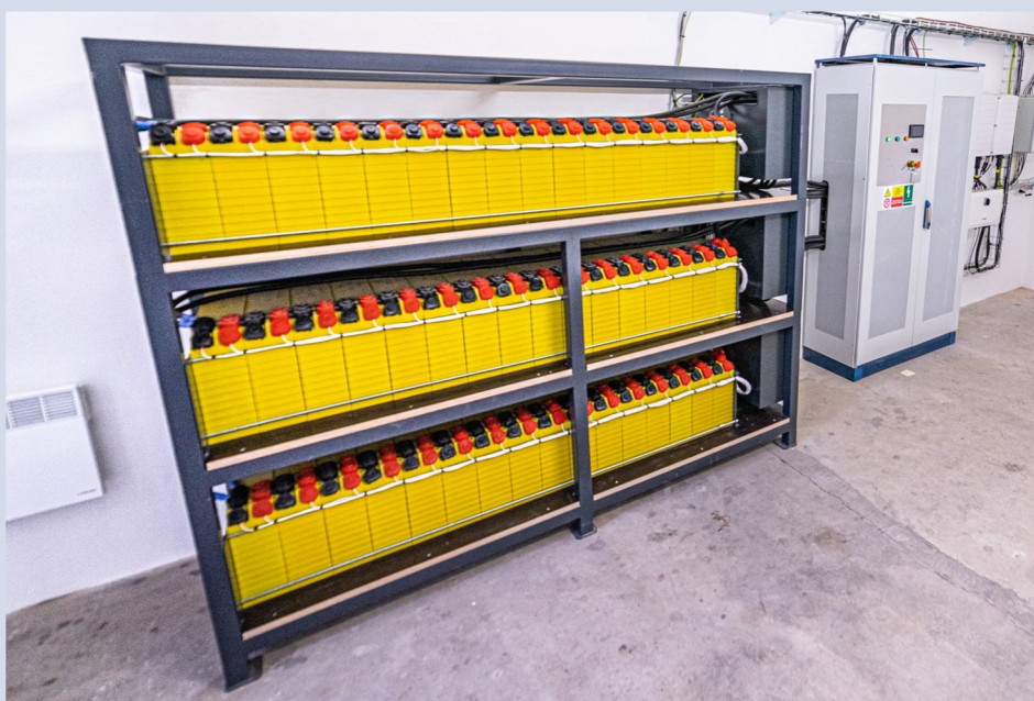
Fig.: 3x AMVOLT 50kWh Module in three floors above each other. 3x16 pieces of LiFePO 4 cells Winston WB-LYP1000AHC 3.3 V, 1000 Ah with nominal voltage 48 V, general installation contractor: ENER-SERVIS a.s. + Tomáš Vocílka (Asolar s.r.o.)
